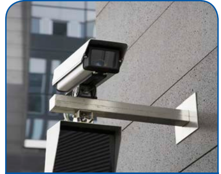
Building Automation & Control
